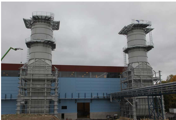
Figure 3 Forssa Power plant commissioned for Fingrid [17].
