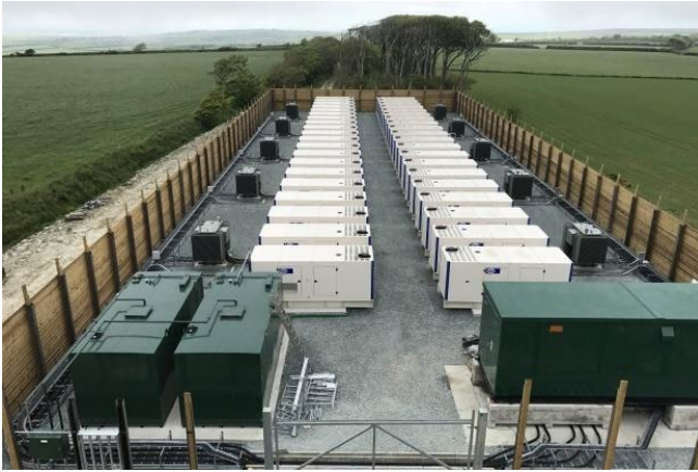
Figure 2 Emergency plant in Cornwall. Photograph: SEA Trasformatore
