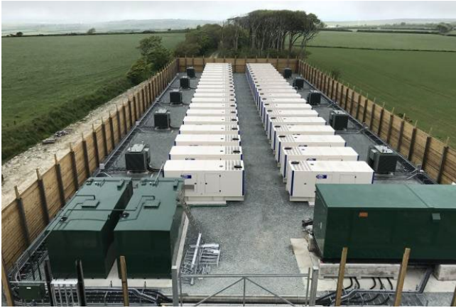
Figure 2 Emergency plant in Cornwall. Photograph: SEA Trasformatori
