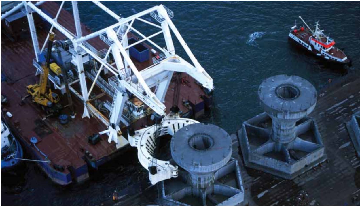
FIGURE 3.7 Photos of the turbine foundations before they were positioned on the seabed.
